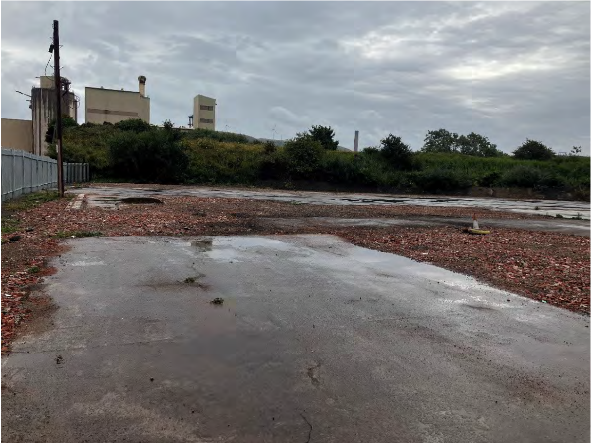
Image EDP A1.17: View east across western parcel of site, illustrating its composition of hard standing, with some evidence of foundations, likely from the late 20 th Century buildings
