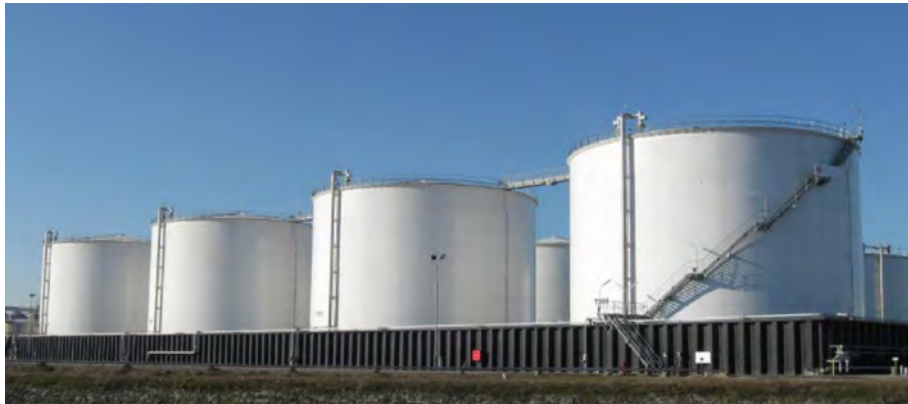
Figure 45 – Typical vessels for the storage of feedstock ethanol in a bunded compound.
