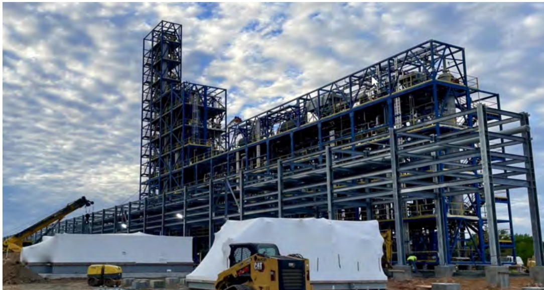
Figures36 – A similar facility to Project Dragon, LanzaJet ATJ plant at Freedom Pines Biorefinery in Georgia, USA is approximately 1/3 the size of proposals in area. Heights of equipment are comparable.
