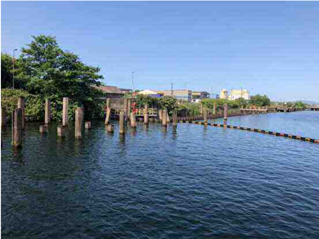
Photograph 10: View from southern site area, facing south-west towards existing cofferdam and remaining stone columns.
