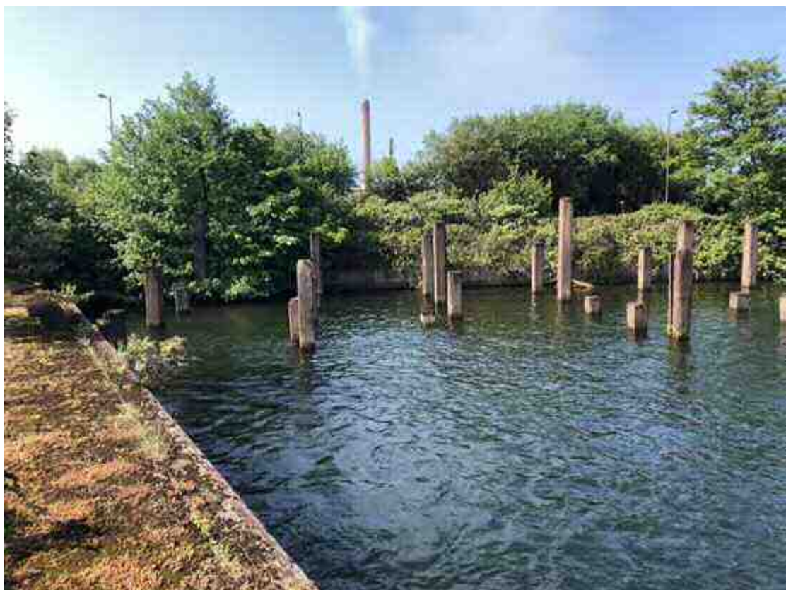
Photograph 12: View from harbour wall, facing south-west towards damaged retaining wall (now covered with dense vegetation) – Photograph taken 25 May 2023.
