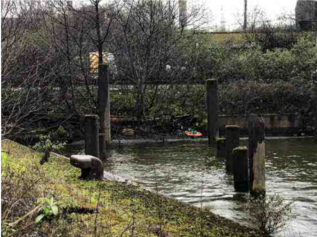
Photograph 11: View from harbour wall, facing south-west towards damaged retaining wall – Photograph taken 29 April 2023.
