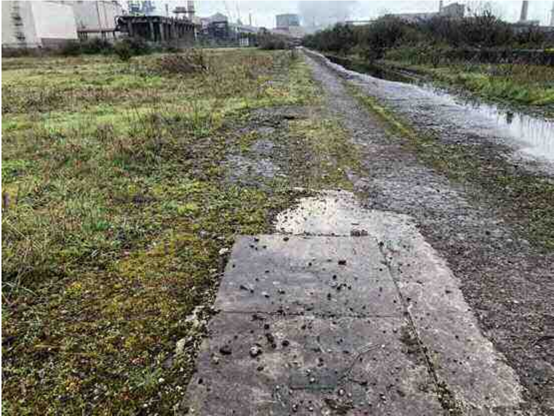
Photograph 4: View facing south, towards BT service cover located parallel to existing access road.
