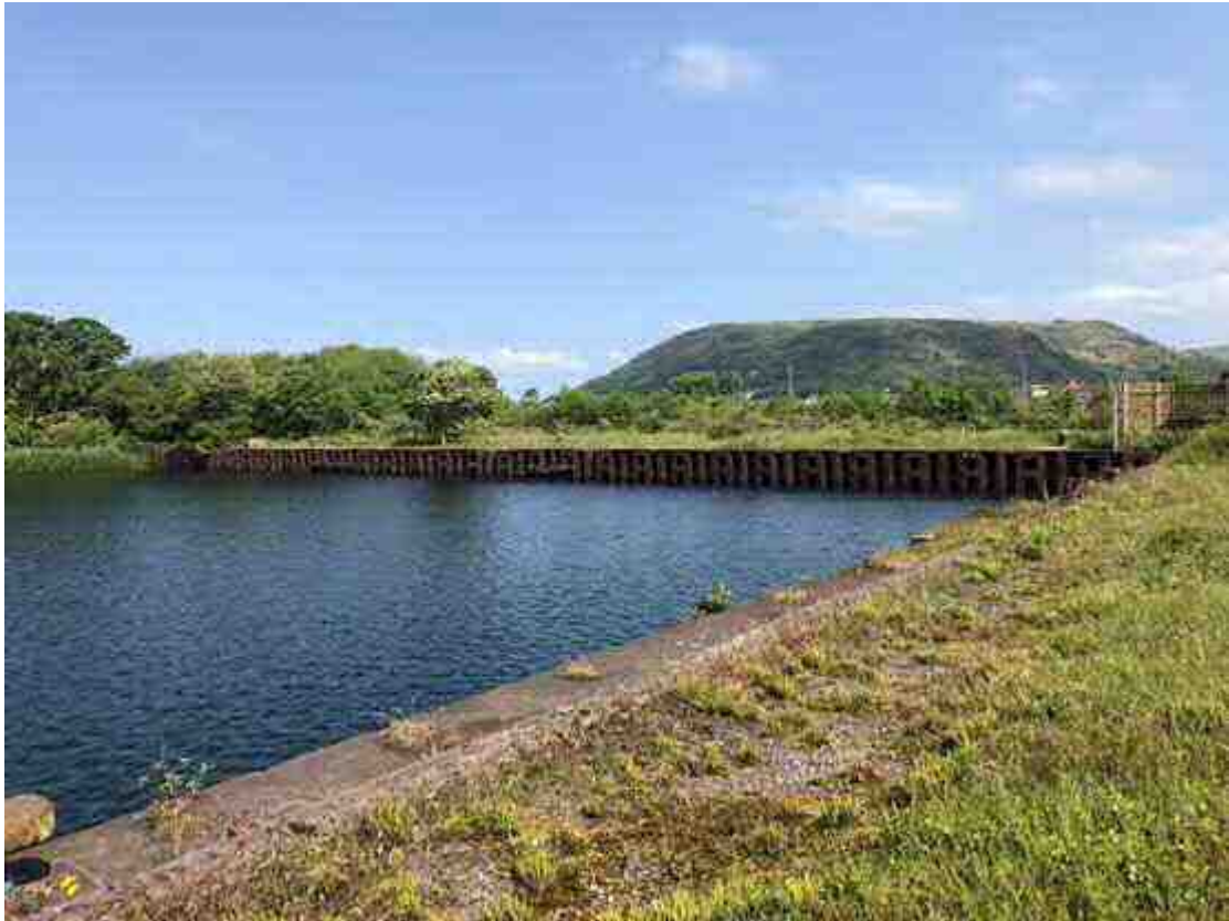
Photograph 7: View facing north-west towards neighbouring harbour wall made up of combined sheet piled wall.
